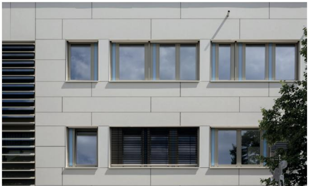
▲ In total, 550m 2 of ultra-compact Dekton by Cosentino surfaces were applied to the facade in the colour Edora
